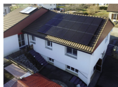
34 m 2 – 6.3 kWc 1727 Corpataux-Magnedens
